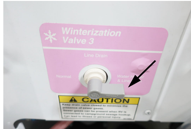
Winterization Valve 3 (Turn it to the Water Heater and Line Drain position). -Typical View
