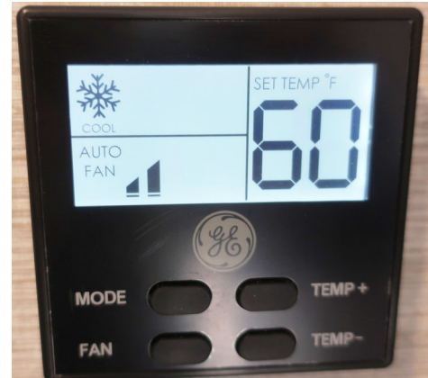
Air conditioner controller (located near the monitor panel) -Typical View
