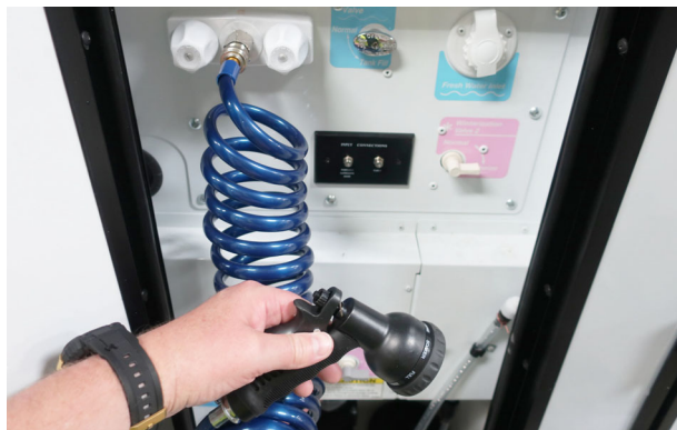
Shower hose shown connected. (Located at Water Service Center). -Typical View
