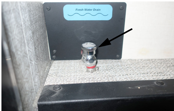
Open and drain the one General Waterline Drain- Passenger Compartment Drain Valve (Shown in the open position). -Typical View
