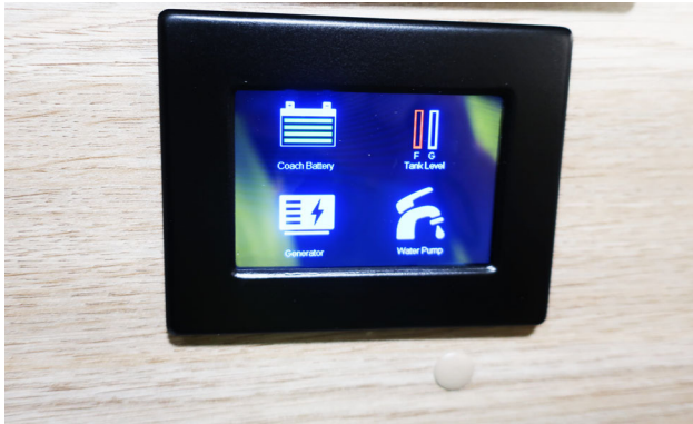
System Monitor Panel -Typical View
