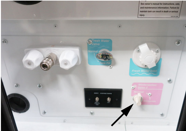
Winterization Valve #2 Located on Water Service Center. -Typical View
