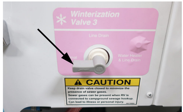
Place the Winterization Valve 3 into the “Normal” position. -Typical View
