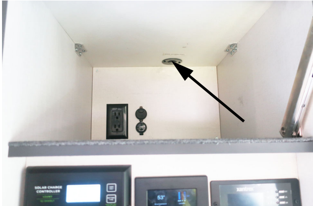
Roof Access Port (Located inside rear overhead cabinet). -Typical View
