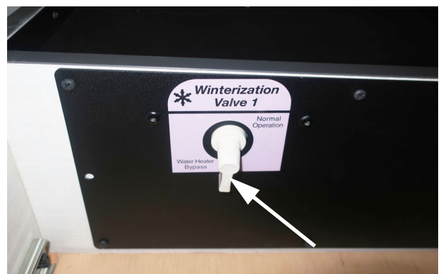
Place the Winterization Valve 1 in the “Water Heater Bypass” position. -Typical View
