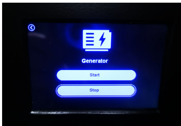
Generator Start/Stop Buttons (Located on the systems monitor panel) -Typical View
