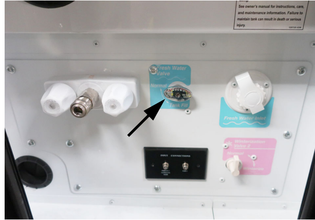
Fresh Water Valve (Drain). (Shown in the closed position). -Typical View
