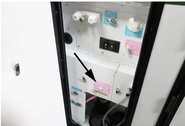
Waterlines Valve #3 Located on Water Service Center. -Typical View
