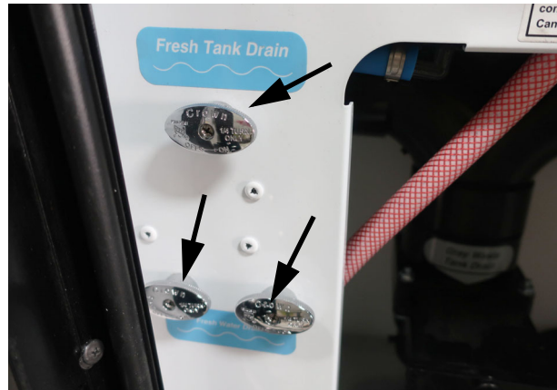
3 of the General Waterline Drain Valves. (Shown in the closed position) -Typical View
